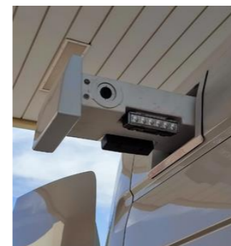
Video surveillance system for recording the objects that caused the alarm
